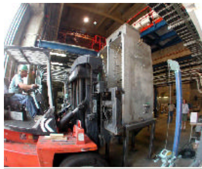
The Modulator enters End Station B, with the crane ready for the next phase of the move.
