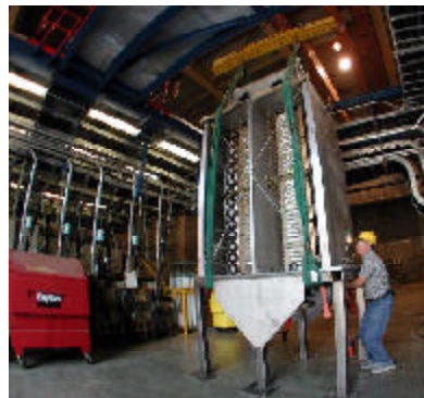
Inside End Station B, the Crane is Ready to Pick Up the Modulator.
